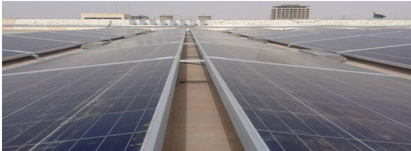
Figure 2. Solar power system installed at Sebha Hospital.
