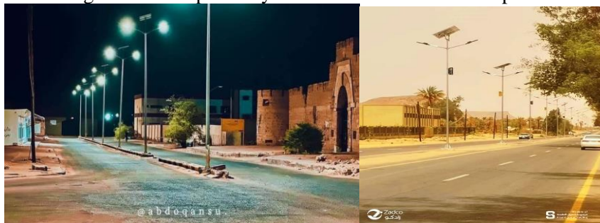
Figure 3. Street lighting using solar panels in Ubari [24].
