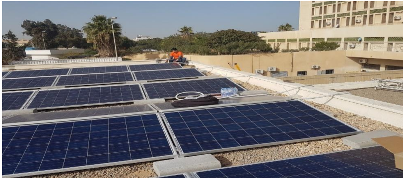
Figure 1. Solar energy system installed at Ubari Hospital.
